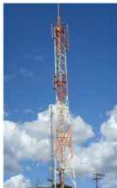
Torre Autoportante (Greenfield)
